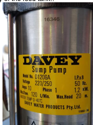
Davey sump pumps installed rated at 120 litres per minute
