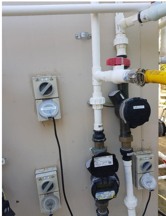
In line cam lock fitting and valve for injection of the additional influent as desired into the line feeding the STS.
