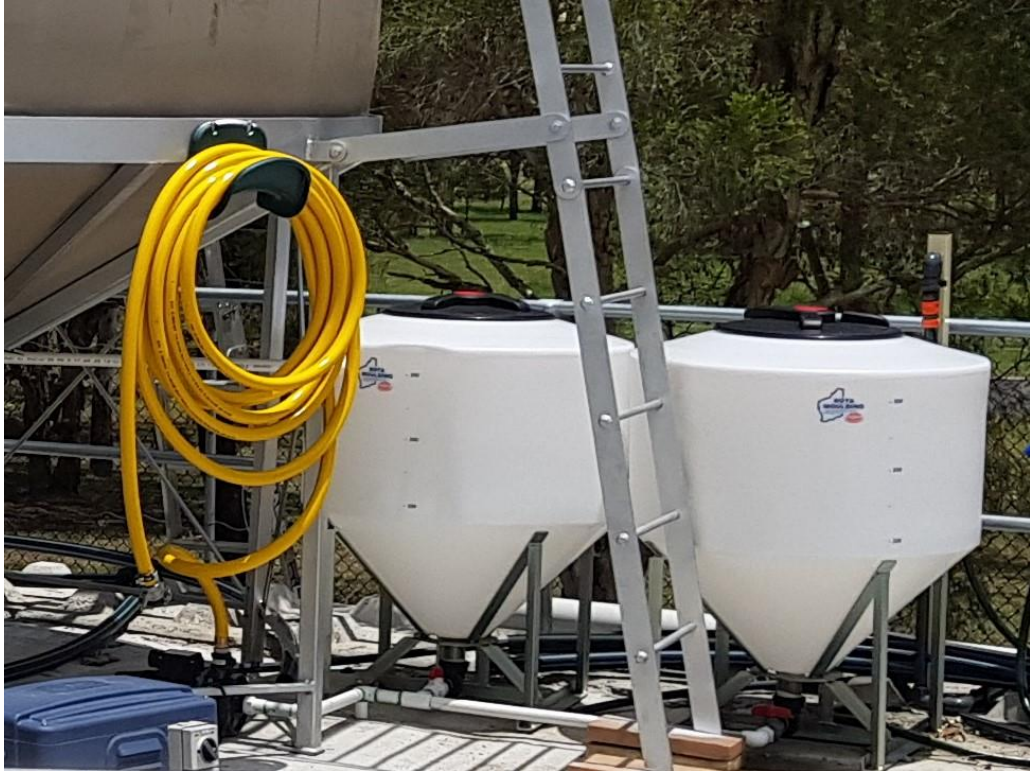
300 litre conical feed tanks, centrifugal pump capable of 100 litres per minute and flexible pipe line with a cam lock fitting.
